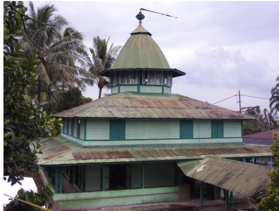
Figure 5. Surau Gadang , Koto Anau, Surau Gadang, Koto Anau, built in 1905 AD, restored in 2008
