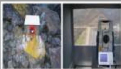
Fig. 10. Sensor installation and data monitoring system.
